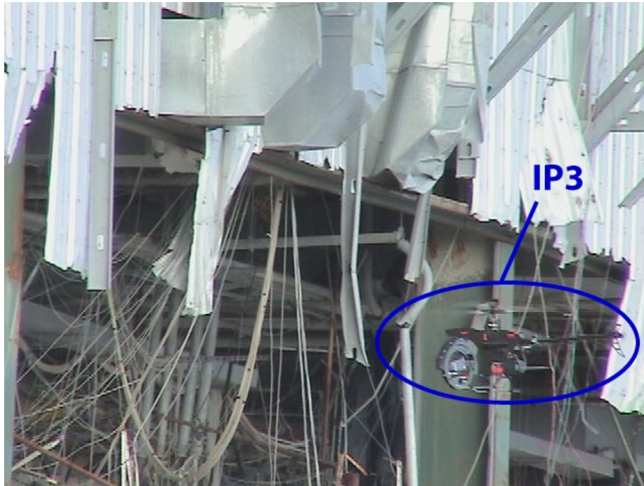
Figure 9: IP3 Hovering in front of a destroyed barge. Radio glitches were a common problem, and a major factor in these was twisted and scattered metal causing multi-path signal interference. Following Figure 1, this provides another example of disaster area obstacles (hanging wires and sheet metal)
